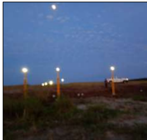
Approach lights installed
