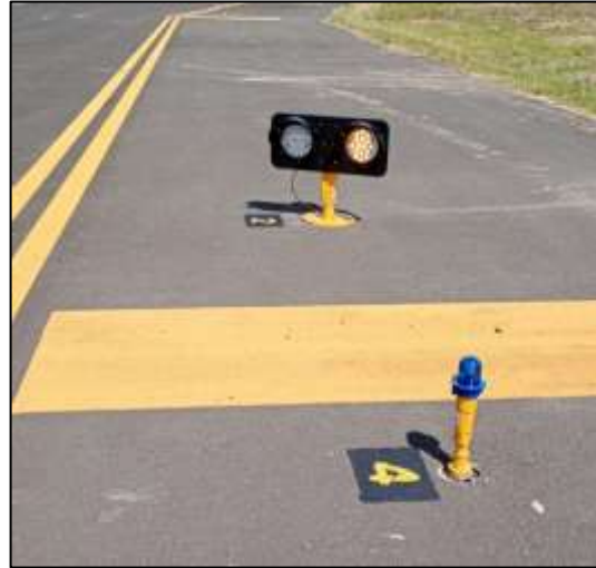
Taxiway and runway guard Lights
